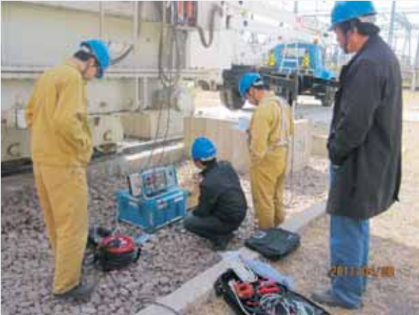
500kV Tranformer Bushing CT
