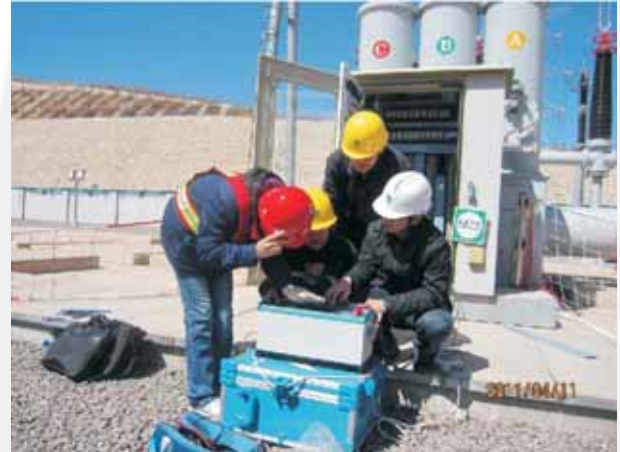
220kV Transmission Line CT
